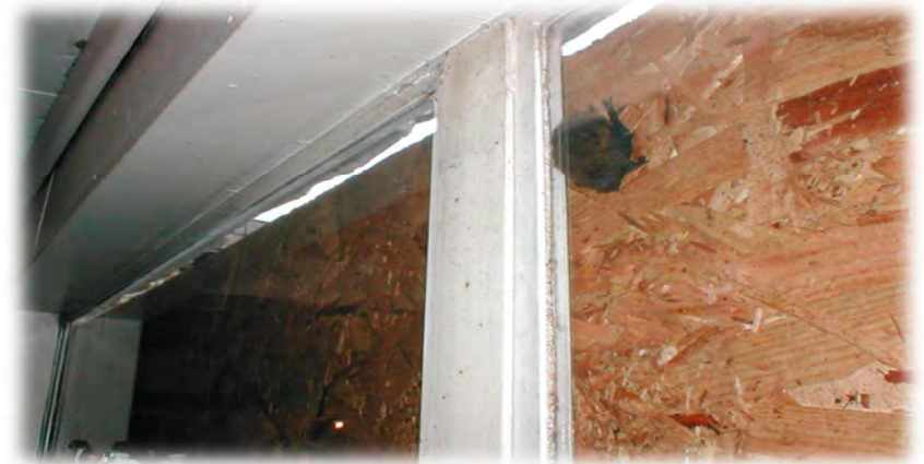
Figure 1: Bat roosting behind boarded-up window
